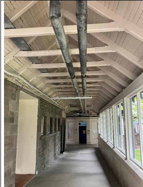
Interior of covered walkway leading from the administration building, looking south towards the octagonal clock tower (31/05/2023) © Historic Environment Scotland
