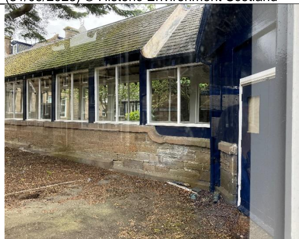
Exterior of the covered walkway showing overhanging eaves and slated roof (31/05/2023) © Historic Environment Scotland
